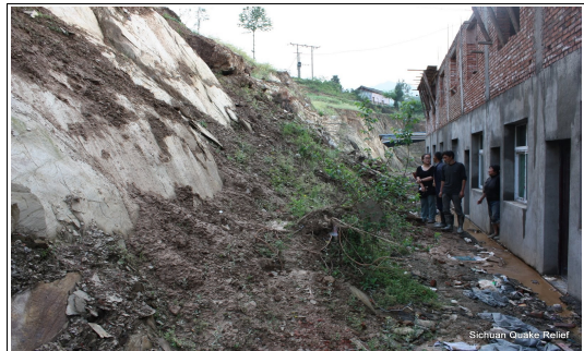
Rainwater washes down this steep, unreinforced slope and collects at the base of unfinished housing in this village in northern Sichuan, permeating the concrete foundations and the floors inside. (May 2010)
